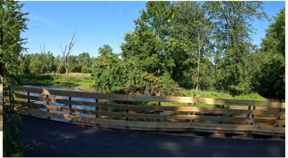
Project TR108 - City of Lansing River Trail Bank Stabilization near Mt. Hope Cemetery
