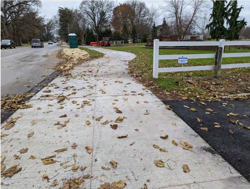
Project TR068 Meridian Township MSU to Lake Lansing Connector, Phase 2b - Okemos Road
